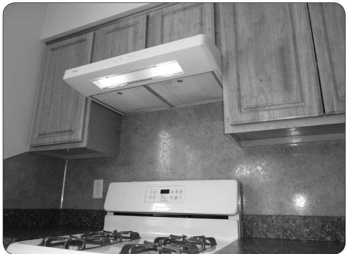
Kitchen exhaust fans remove moisture from the air, which prevents mold growth and other related problems that can occur from excess water vapor.
